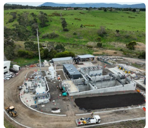
Gisborne Recycled Water Plant
