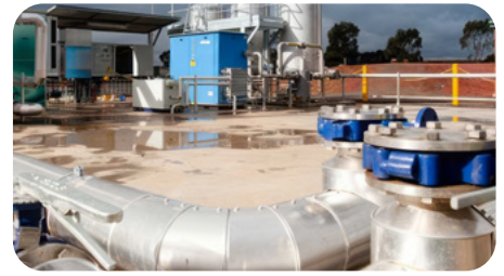
Our Melton Recycled Water Plant
