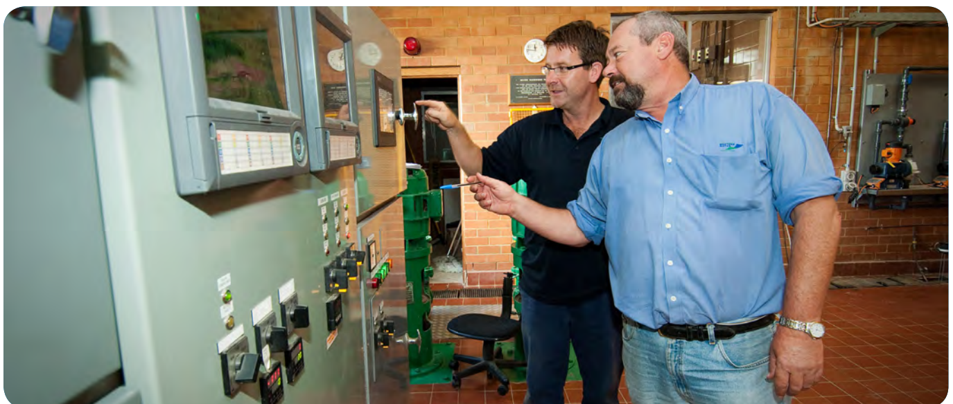
Water quality system monitoring, Merrimu Water Filtration Plant
