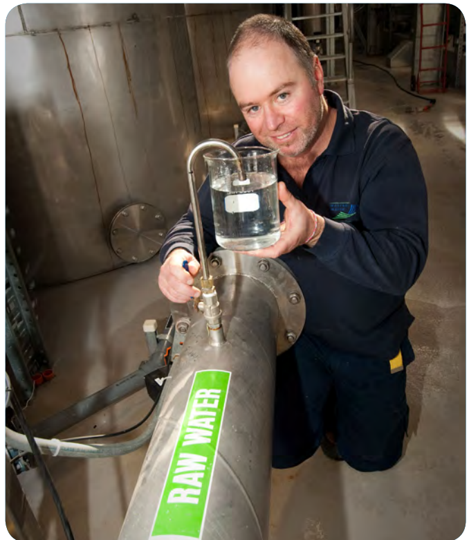
Water quality monitoring, Lancefield Water Filtration Plant
